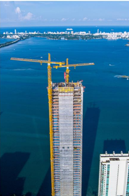
Missoni Baia in Miami has topped out at 57 stories and 198 meters. Image credit: Golden Dusk Photography
