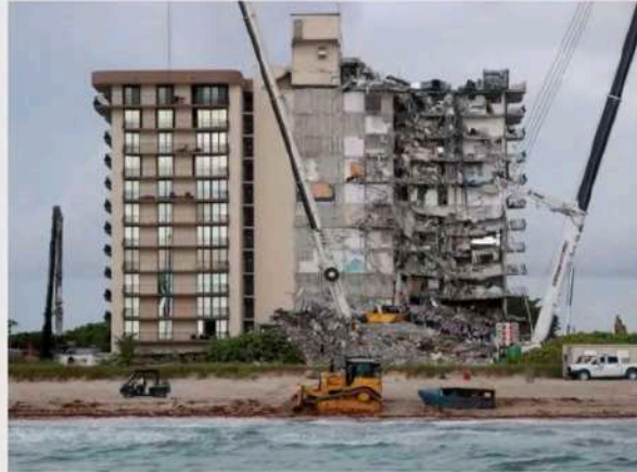
Champlain Towers South collapsed more than two years ago. Investigators say the condo’s concrete columns and pool deck were constructed improperly and its steel was corroded.
